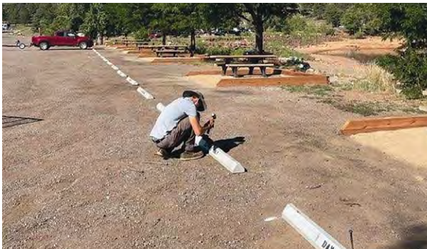
Bottom left: Setting parking stops ensures visitors know where to go when visiting a day use area.
