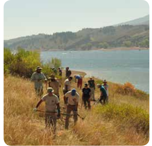
Volunteers assist Larimer County staff with constructing a new section of the Foothills Trail last fall at Horsetooth Reservoir. Photo © Zach Schierl
