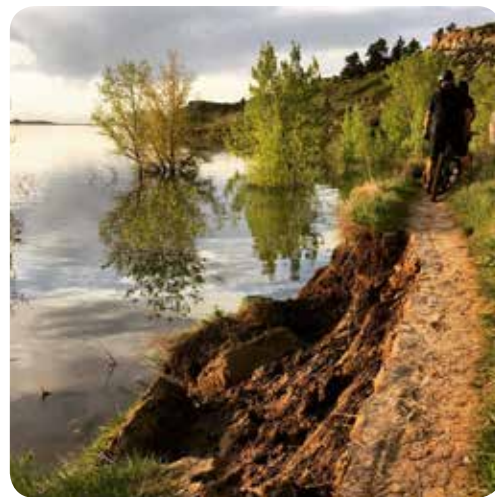
A wet spring with high water levels at Horsetooth Reservoir led to the collapse of a section of the Foothills Trail. Photo © Josh Weinberg
